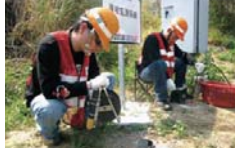
邊坡監測 | Slope Monitoring
