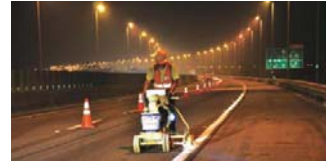
標線施設 | Marking Traffic Stripings
