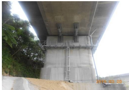
Figure 14: STUs and maintenance catwalk
